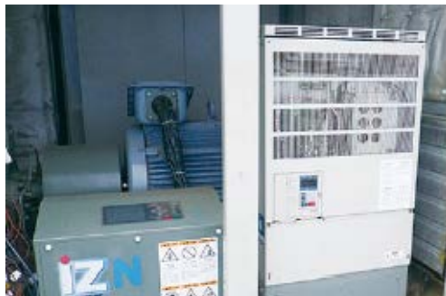
Refrigeration Equipment Using Natural Refrigerants (ammonia)
