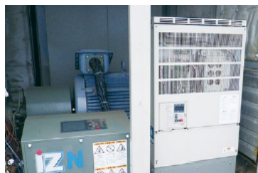
Refrigeration Equipment Using Natural Refrigerants (ammonia)
